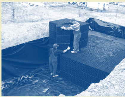
Underground tank and pump
