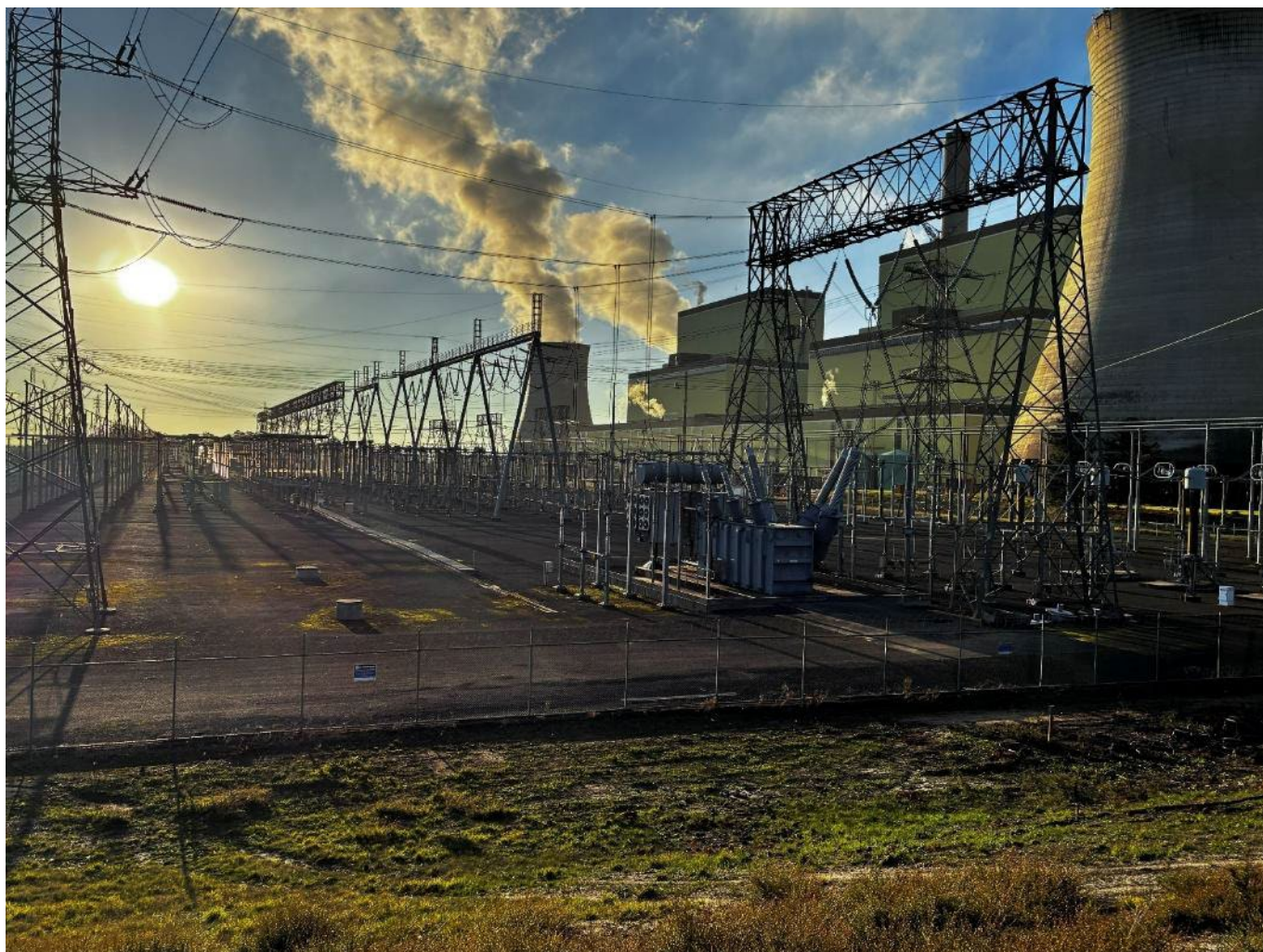
Plate 2 View of switchyard facing west
