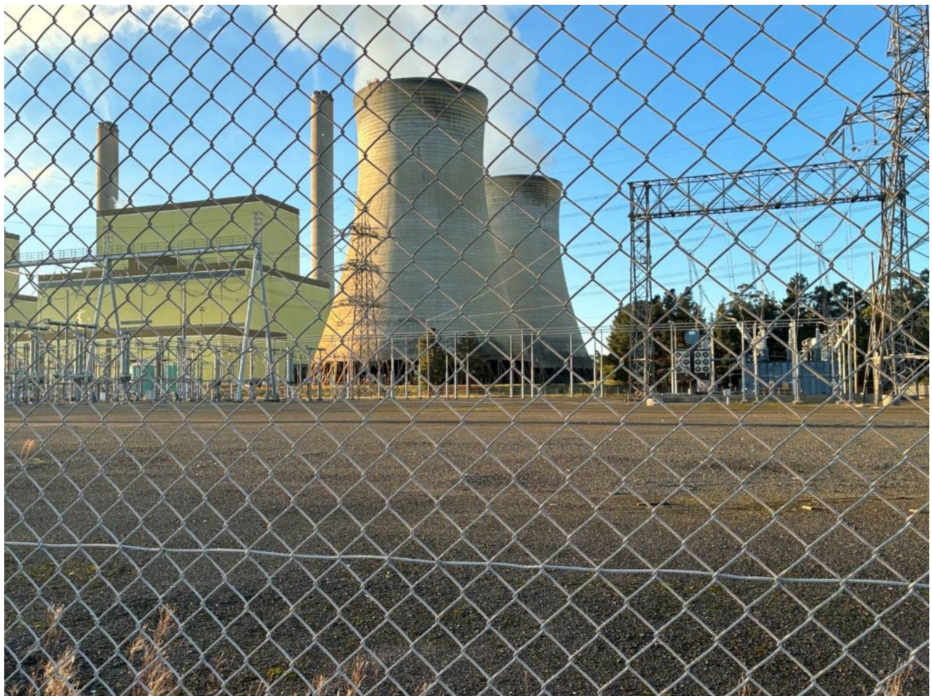
Plate 1 Location within switchyard where the proposed Bay 17 and Bay 18 would be installed
