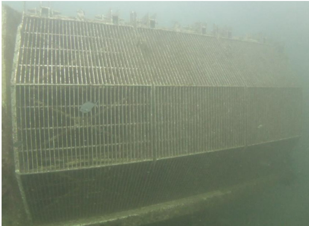
Figure 7. Seawater intake grille at Victorian Desalination Plant (Photo by M Venturoni)
