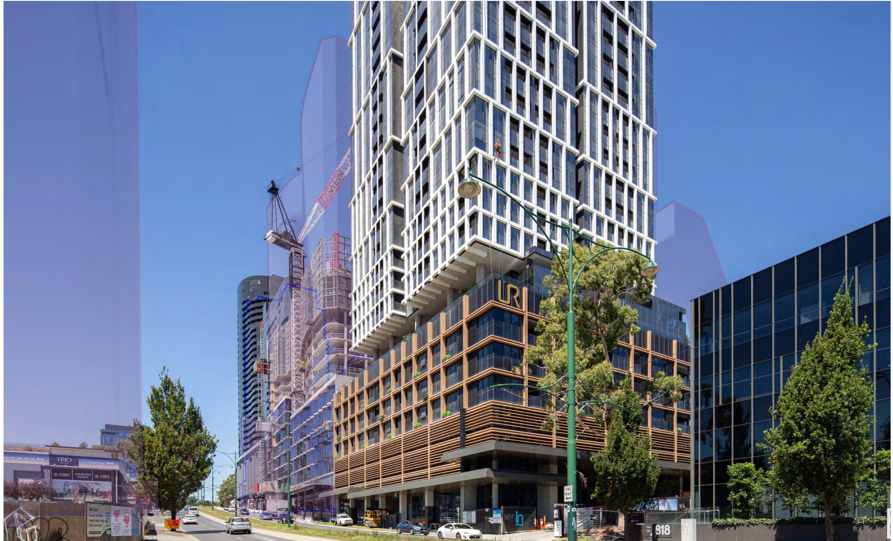
/View 4 - From corner of Poplar Street and Whitehorse Road to west of the MAC
