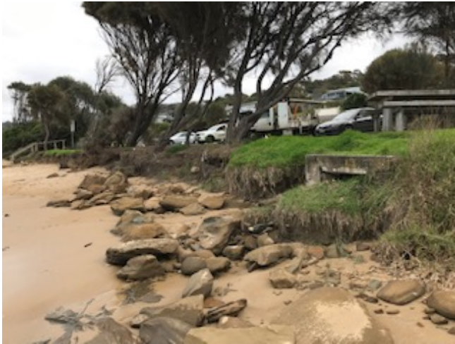
Picnic area erosion July 2019
