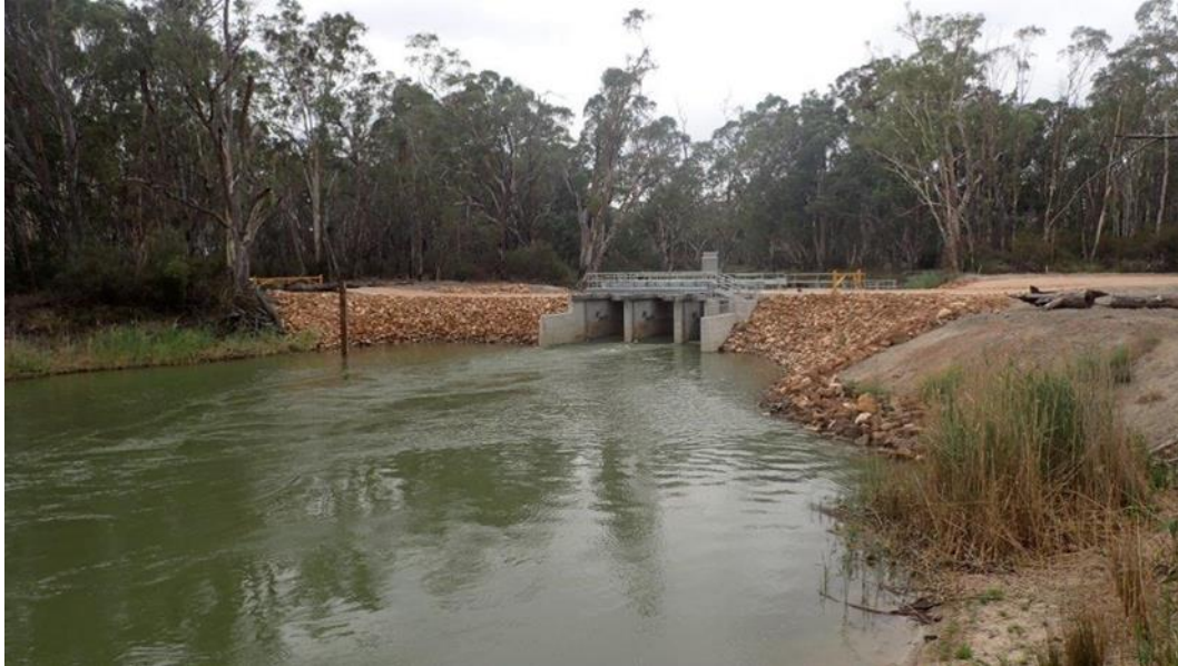
Figure 1 – A regulating structure at Mullaroo inlet, similar to the K10 regulator proposed
