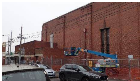
Figure 3-26 View of the substation and shopfront attached to the tram shed (note cherry picker), facing southeast
