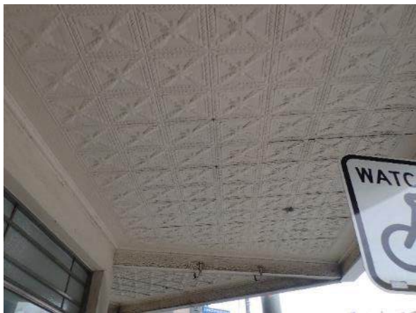
Figure 83. View of the moulded tin panels under the shopfront awnings, facing north
