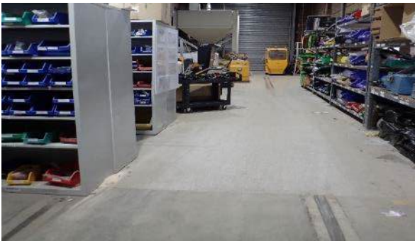
Figure 3-22 View of Roads1, which has been filled in, inside the former wheel grinding workshop, facing west
