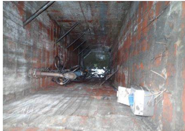
Figure 3-11 View down into the brick-lined well, with ladder rungs and piping, and water at the base
