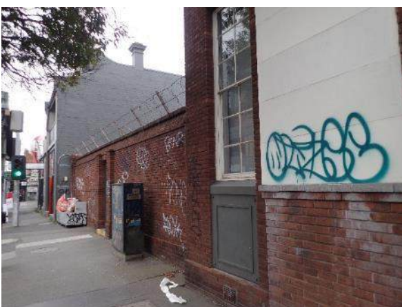
Figure 54. View of wall between the Traffic and Revenue office building and the adjacent building, facing southwest
