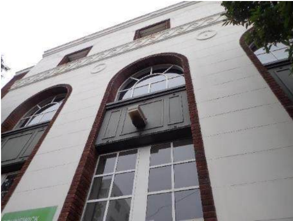
Figure 56. View of wall between the Traffic and Revenue office building and the adjacent building, facing southwest
