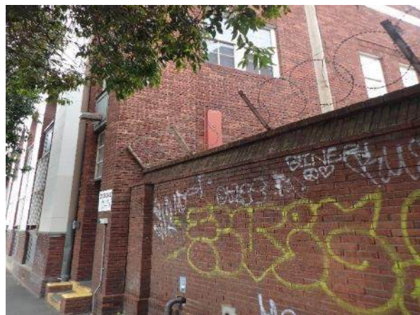
Figure 53. View of wall between the Traffic and Revenue office building and the tram shed, facing southwest
