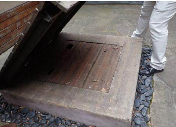
Figure 64. Close up of well with metal covering under timber seating, facing west
