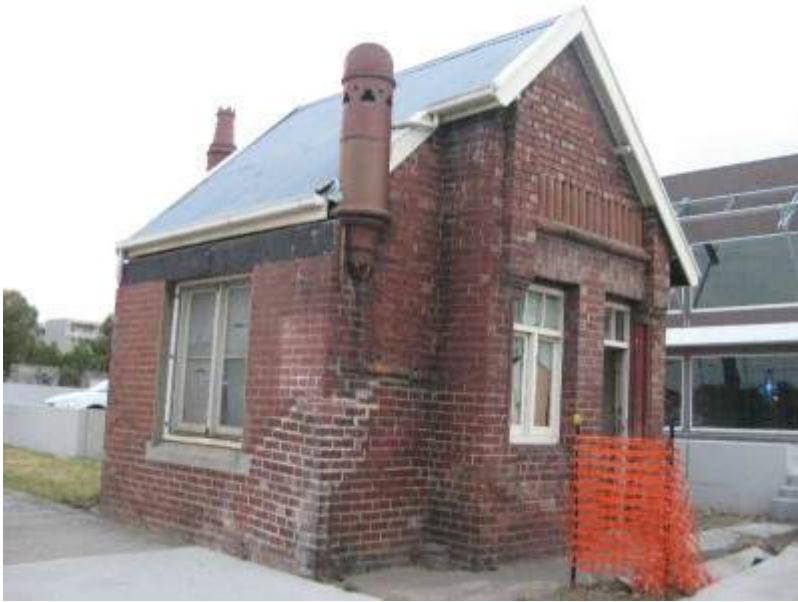
Former Ferry Terra Cotta & enamel brickworks office albert Street brunswick from the northweat
