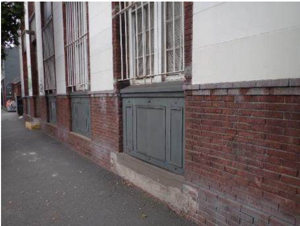
Figure 3-7 View of wall between the Traffic and Revenue office building and the tram shed, facing southwest
