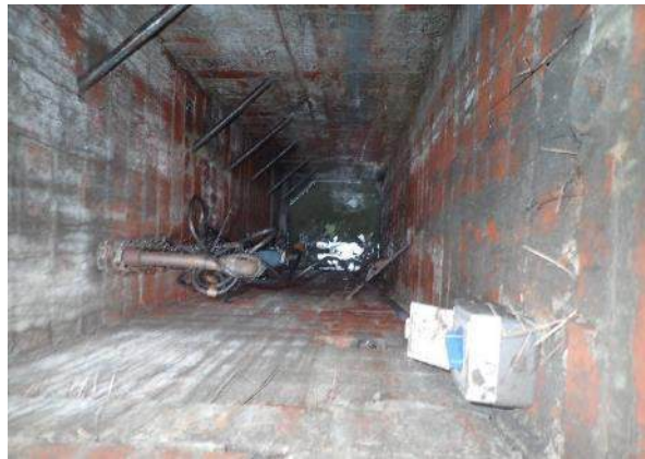
Figure 65. View down into the brick-lined well, with ladder rungs and piping, and water at the base
