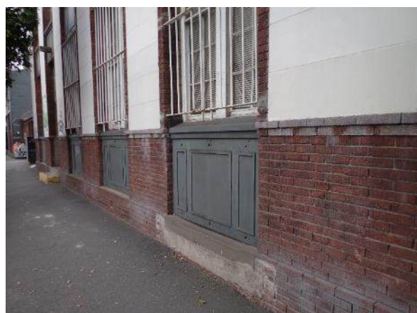
Figure 55. View of wall between the Traffic and Revenue office building and the tram shed, facing southwest
