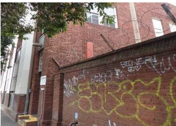
Figure 3-5 View of wall between the Traffic and Revenue office building and the tram shed, facing southwest
