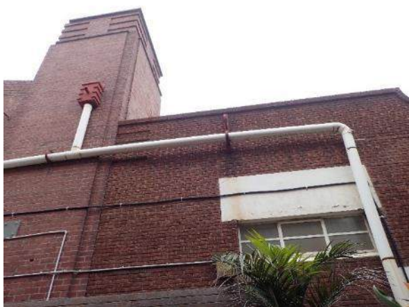
Figure 85. View of the south facing of the shopfront attached to the tram shed and adjacent wall, facing north
