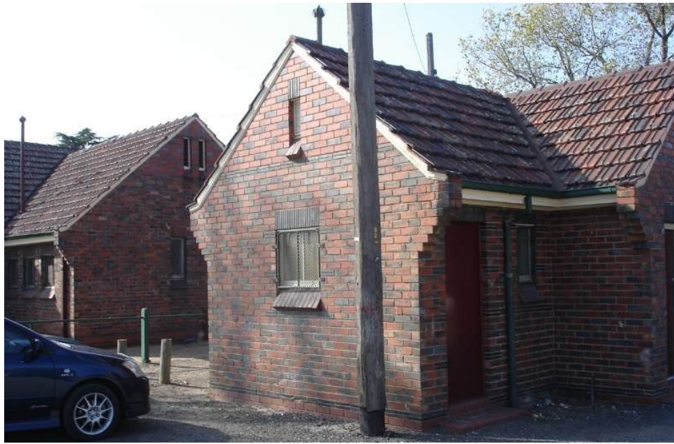
Figure 59. Women's Dressing Pavilion, showing architectural detail. (Source: Victorian Heritage Database, accessed 16 November 2023)
