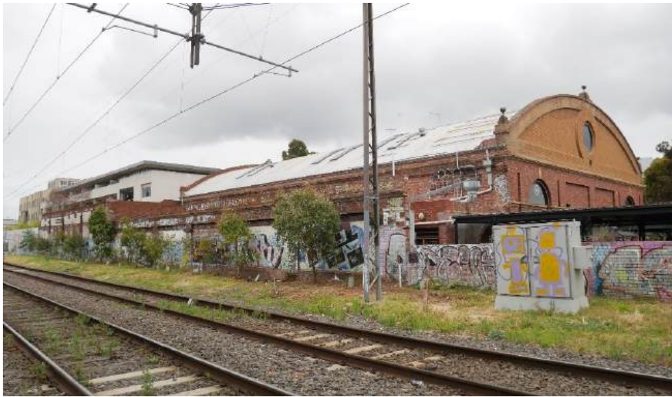
Figure 66. Looking southwest from Hope Street level crossing across the rail corridor to the Former Brunswick Gas & Coke Co Retort House, also showing east boundary wall.
