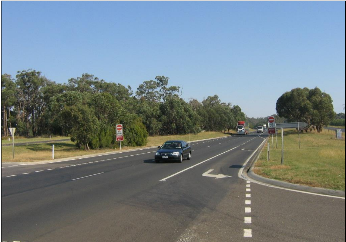
Figure 7 - Princes Freeway at its intersection with North Garfield Road, sealed good condition
