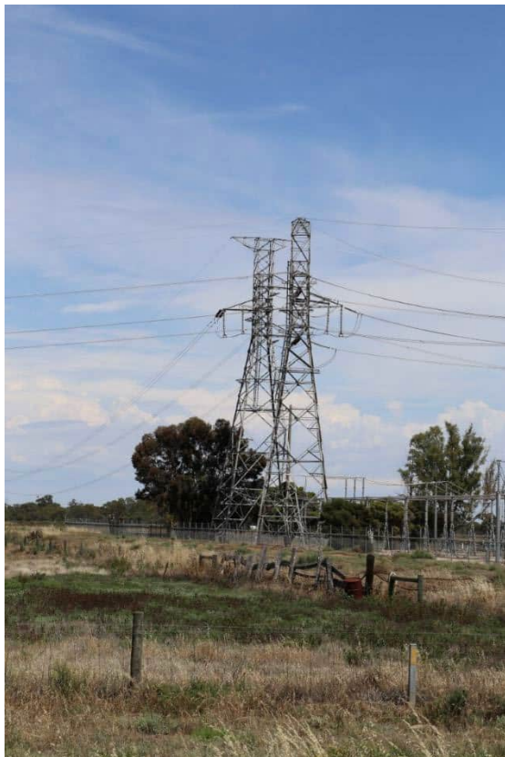
Figure 18 - HV Powerlines connecting to the Kerang Terminal Station traverse the landscape to the west of the Project Area.
