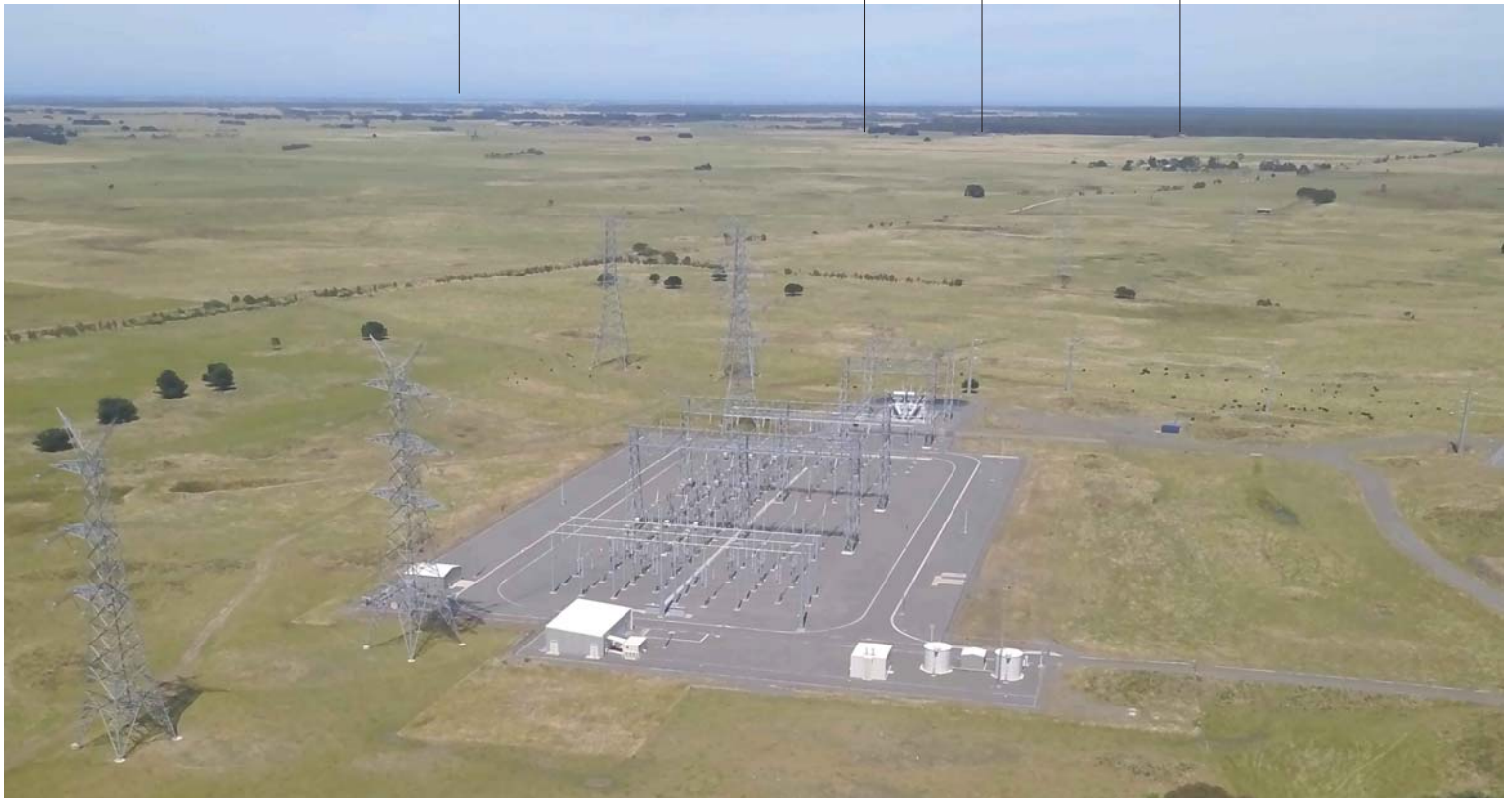
View west to south west from Tarrone substation (west of Tarrone North Road) Kangertong Road looking toward distant views of the Codrington and Yambuk Wind Farm sites
