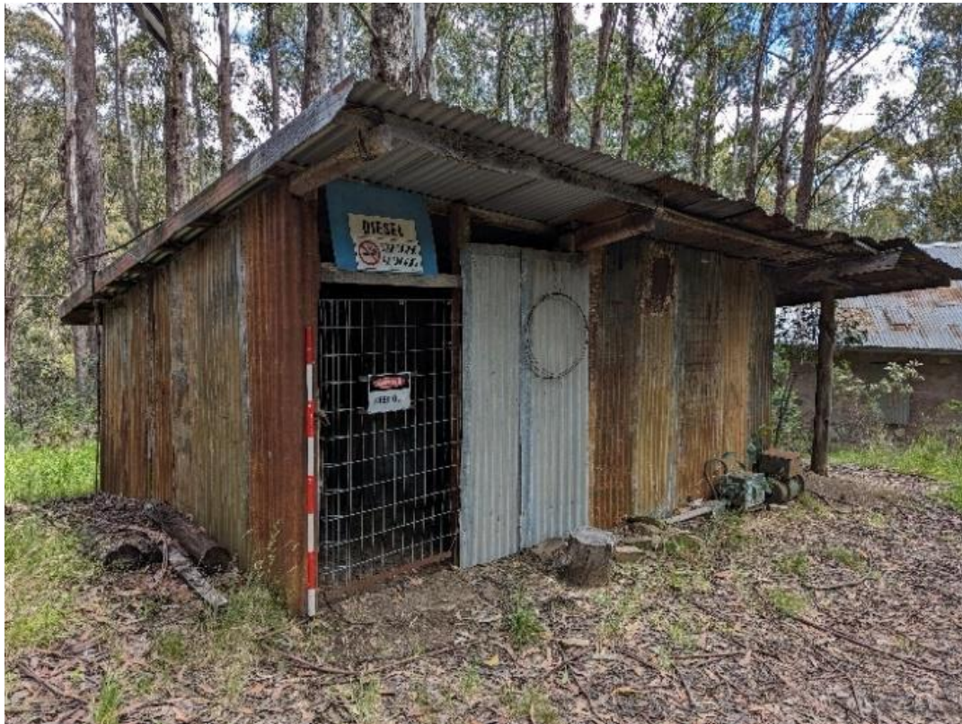
Figure 24. Generator plant and storage shed, located behind the two-storey dwelling.
