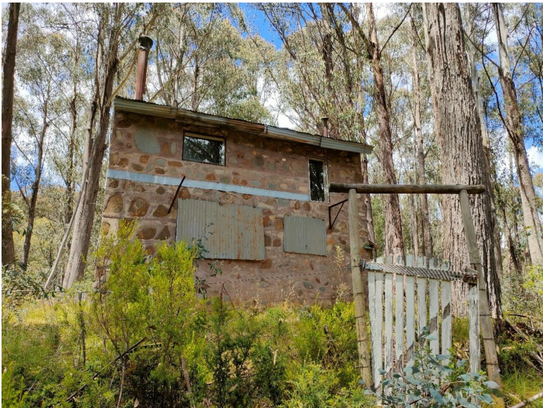
Figure 22. Rear exterior wall of the two-storey dwelling with lower windows covered in corrugated iron.
