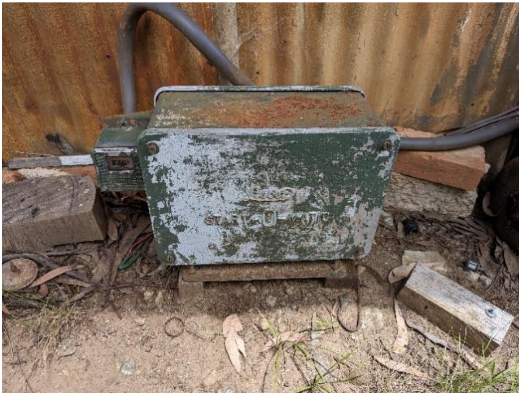
Figure 26. Lister Start-o-Matic generator, as seen outside the shed in the previous figure.
