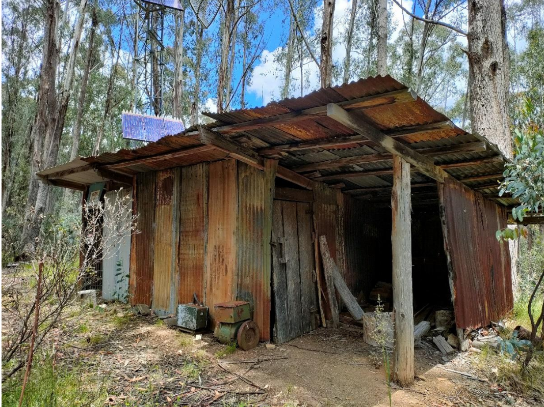
Figure 25. Generator plant and storage shed, located behind the two-storey dwelling.
