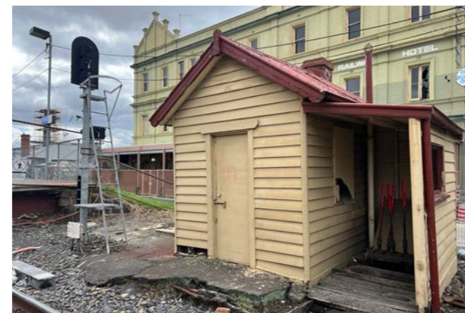
Image 28 Gatekeeper's cabin, which is part of the heritage elements located on the station precinct
