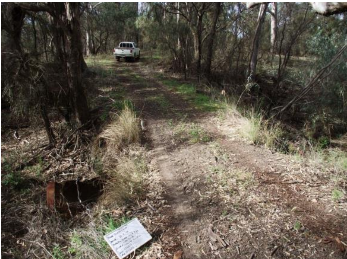
Figure 17: Existing pump diversion block Bank 5 to be modified by the project
