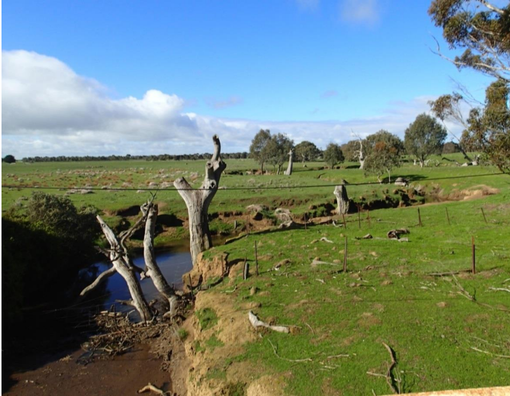
Figure 7 – Degraded section of Kuruc A Ruc Creek (also referred to as Meadows Creek) incised through alluvial floodplain (East of Meadows Road). Source: Jacobs
