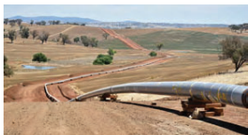
Example of a pipeline under construction, prior to being lowered into the ground.
