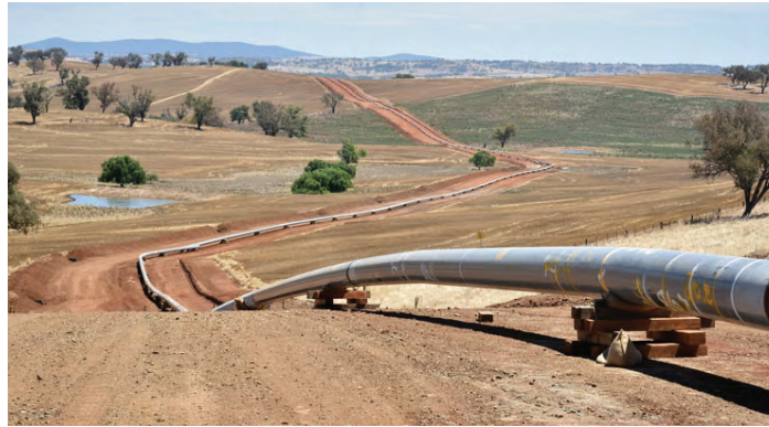
Example of a pipeline under construction, prior to being lowered into the ground.
