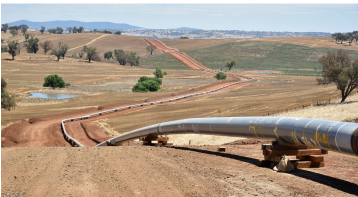
Example of a pipeline under construction, prior to being lowered into the ground.
