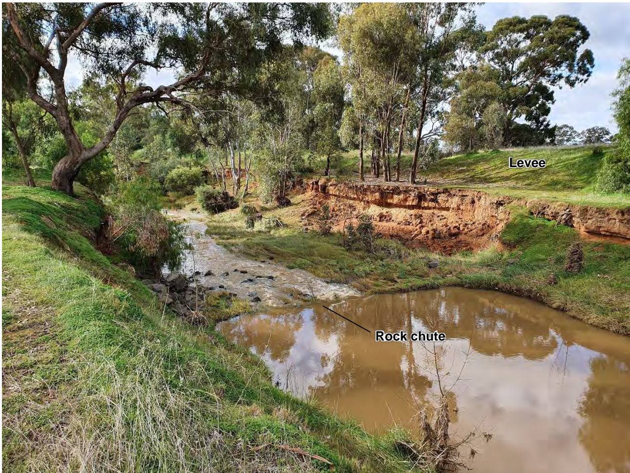
FIGURE 3-10 DOWNSTREAM VIEW OF THE ROCK CHUTE. WHILST IN POOR CONDITION THE STRUCTURE PROVIDES LONGITUDINAL BED GRADIENT CONTROL.
