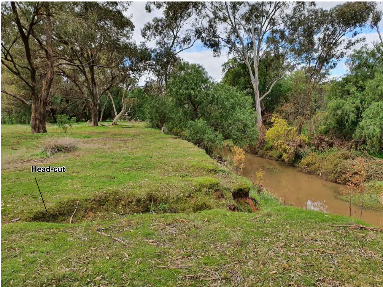
FIGURE 3-5 AN EXAMPLE OF A HEAD-CUT OCCURING INTO THE FLOODPLAIN IN RESPONSE TO DEEPENING WITHIN THE TRUNK STREAM.
