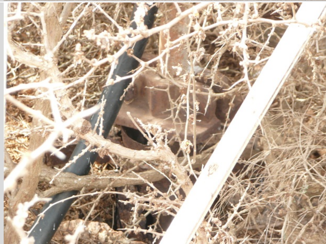
12. Close-up view of mill and bore casing (steel).
