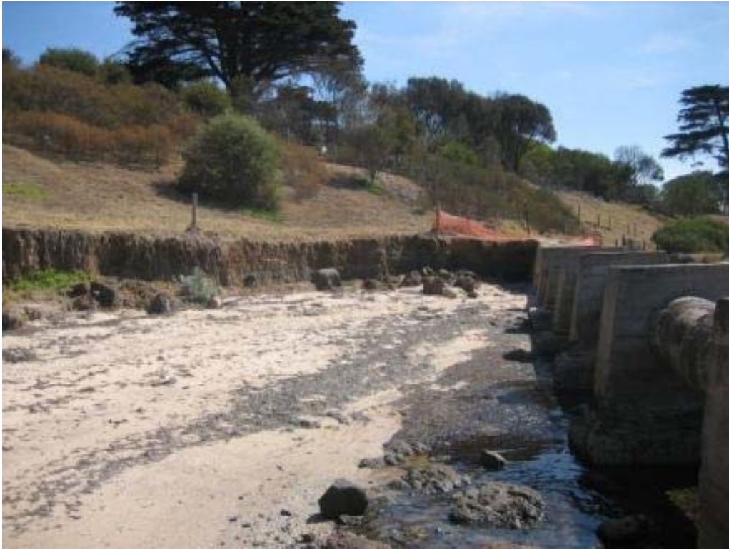
Figure 2-10 Recent Erosion and Undermining of Stormwater Drain Outfall
