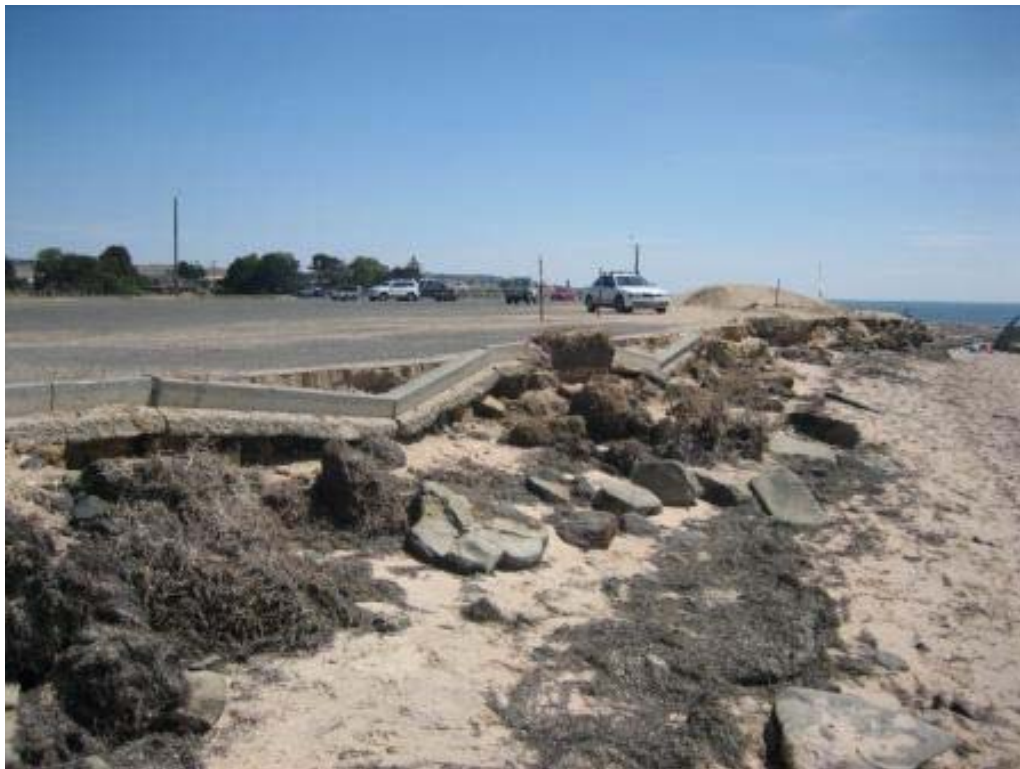
Figure 2-13 Recent Erosion of the Beach along Point Richards
